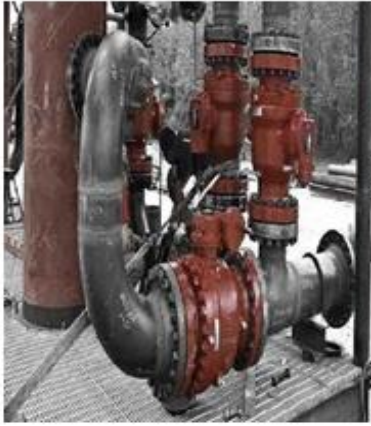
Valves on a manifold
