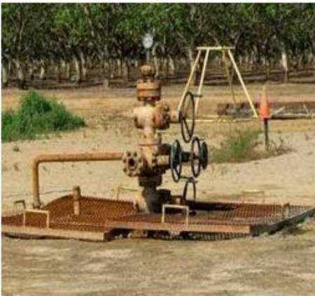
Christmas Tree structured on valves
